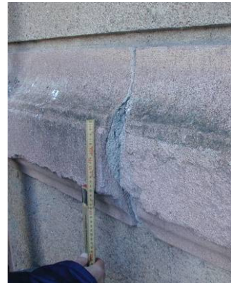
C Gaps in joints between cement elements
