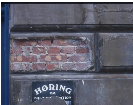
A Flaking of plaster layers
